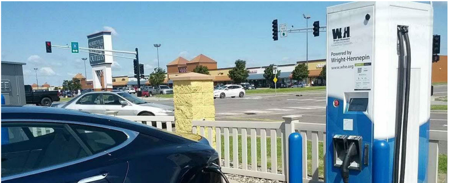
Electric vehicle charging stations provide customers with more sustainable options to access local businesses.
