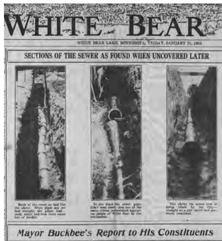
A headline and three photos on the front page of the January 10, 1936 issue of the White Bear Press reminded residents of the many problems the city encountered when its sewer system was installed. The photo on the left shows sewer pipes that were not laid straight, which caused them to leak at the joints. The middle photo shows pipes that were not joined at all. The final photo shows the pipes after they were relaid by city workers. Photo courtesy of the Minnesota Historical Society.
