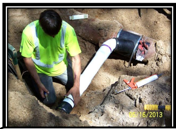
Service 'wye' connection and up to 10 feet of service pipe are replaced during Upcoming construction project
