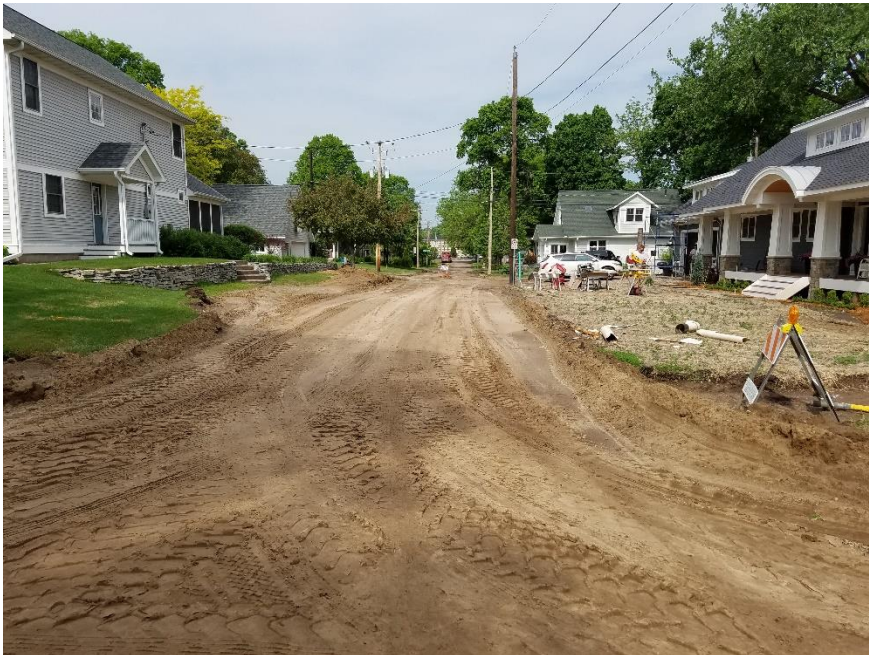
On 9 th Street (viewed westward from Johnson Avenue), deep sanitary sewer repairs were completed at this location over the last week.
