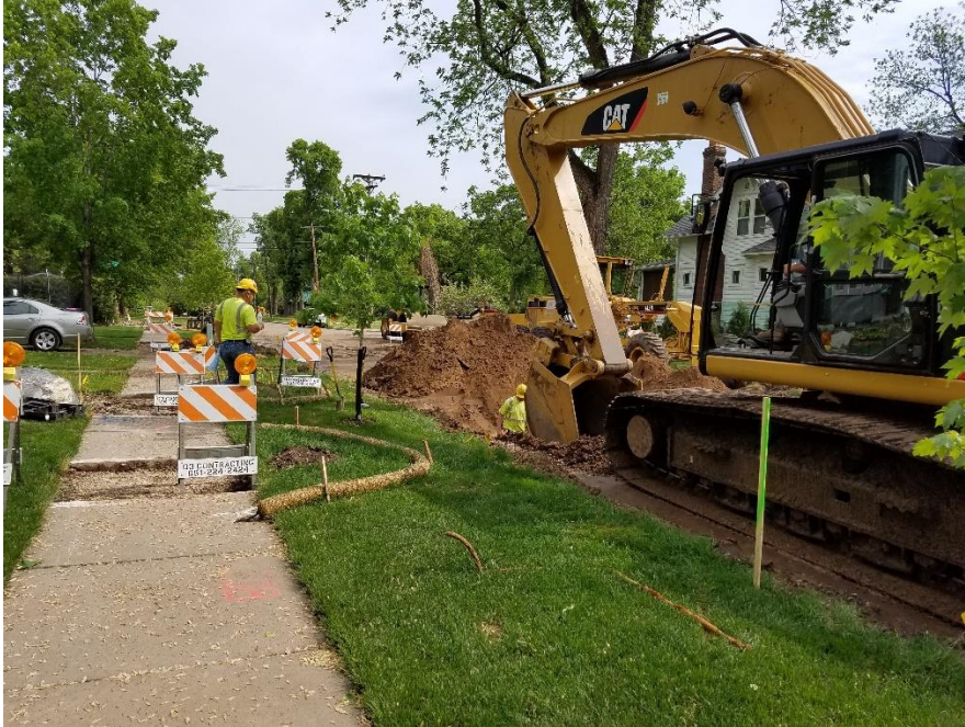
On Johnson Avenue, workers dig to evaluate the material type of the existing water service. Lead and galvanized water services are being replaced with copper.
