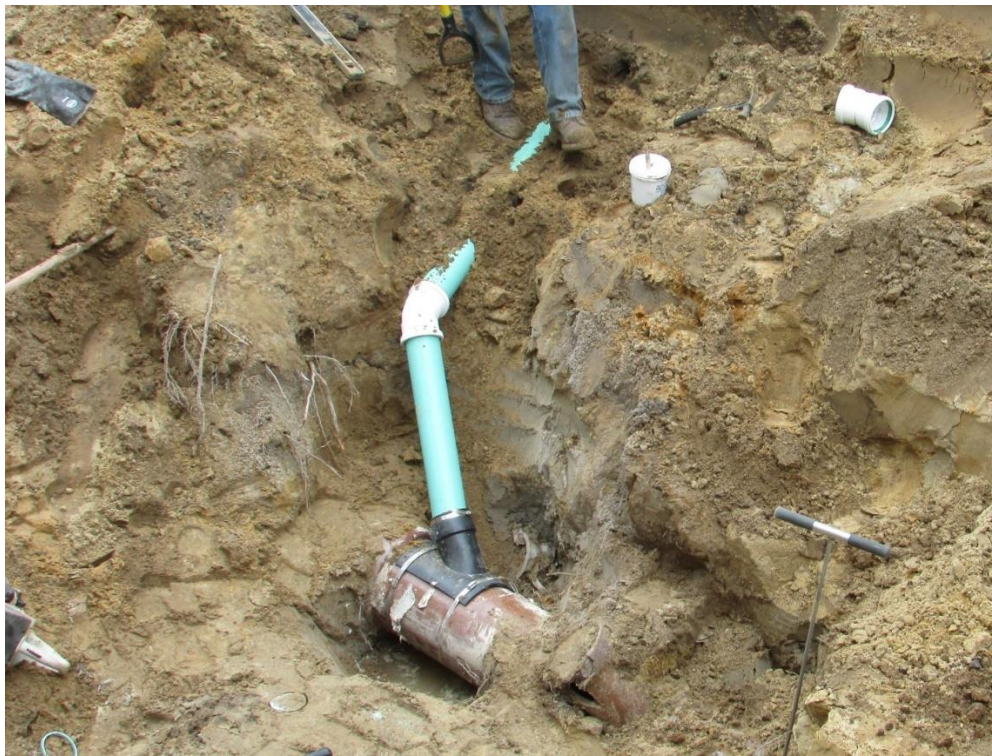
Where necessary, property owners are having their sanitary sewer connection replaced with a new PVC pipe.
