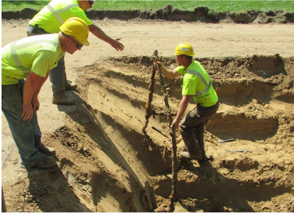
A worker removes an old water service. Brittle galvanized water services are being replaced with copper water services.
