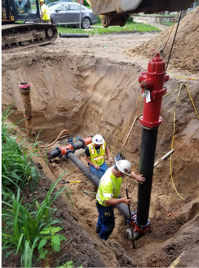
Workers carefully place a new hydrant at the corner of 8 th Street and Morehead Avenue.
