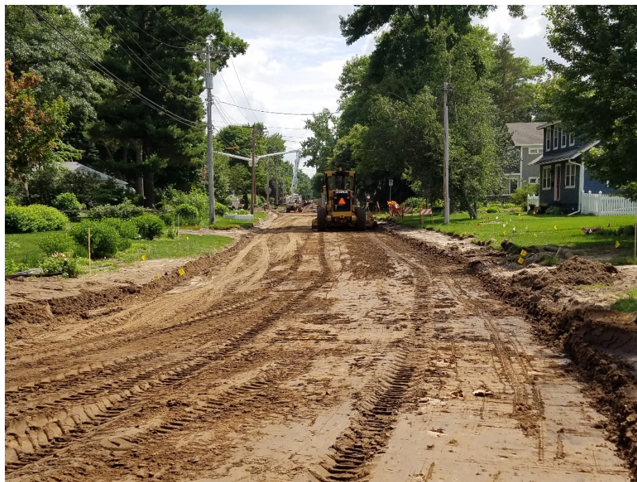
Morehead Avenue looking south from 10 th Street. The street base was cut down earlier in the week and built back up on Friday using specifically sized gravel aggregate.
