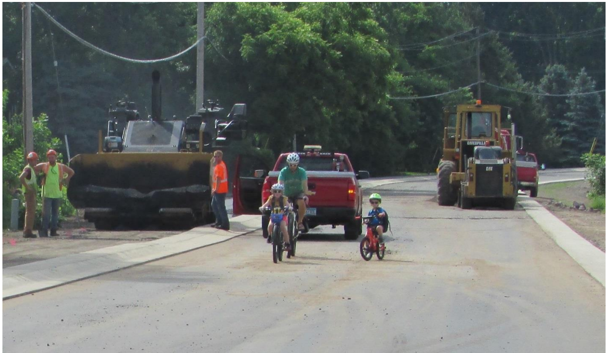
Workers pave the new trail alongside Old White Bear Avenue. Residents and visitors alike are excited about the ongoing trail improvements in the City of White Bear Lake.
