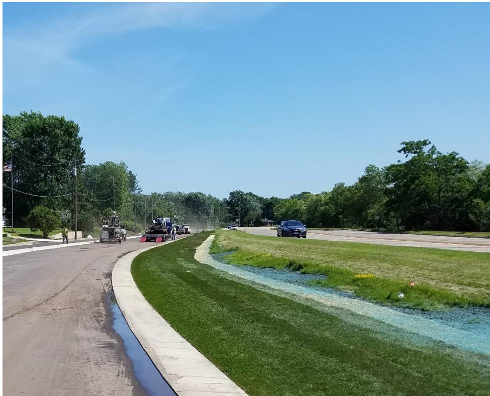
Workers place sod and hydroseed alongside Old White Bear Avenue. This section of Old White Bear Avenue will be seeded with a special native mix of pollinator-friendly plants.
