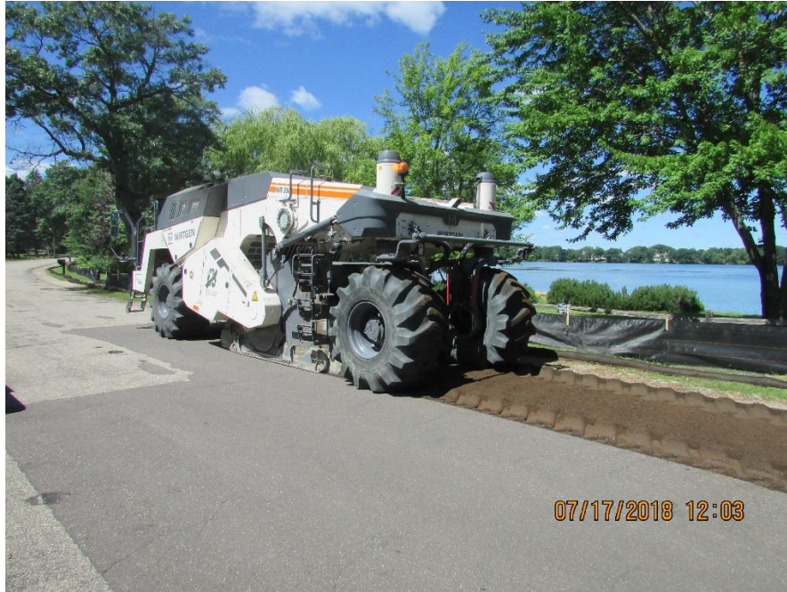
Reclaiming machine the Contractor used to crush the existing pavement into gravel that we will use as a road base.
