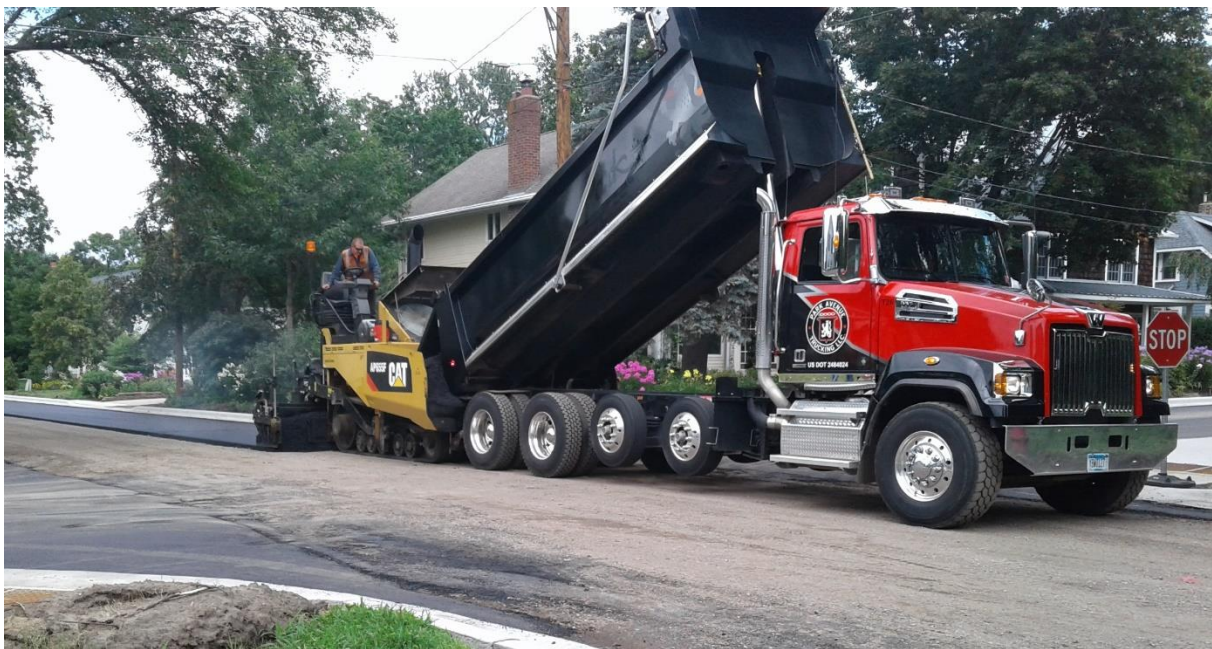
The first layer (base course) of asphalt being placed on Johnson Avenue. Asphalt is placed in layers in order to achieve a superior final product.
