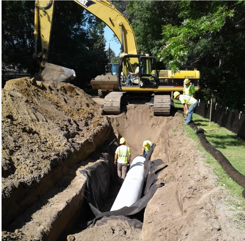
Forest Lake Contracting workers carefully install new reinforced concrete pipe storm sewer at Birch Lake Boulevard South
