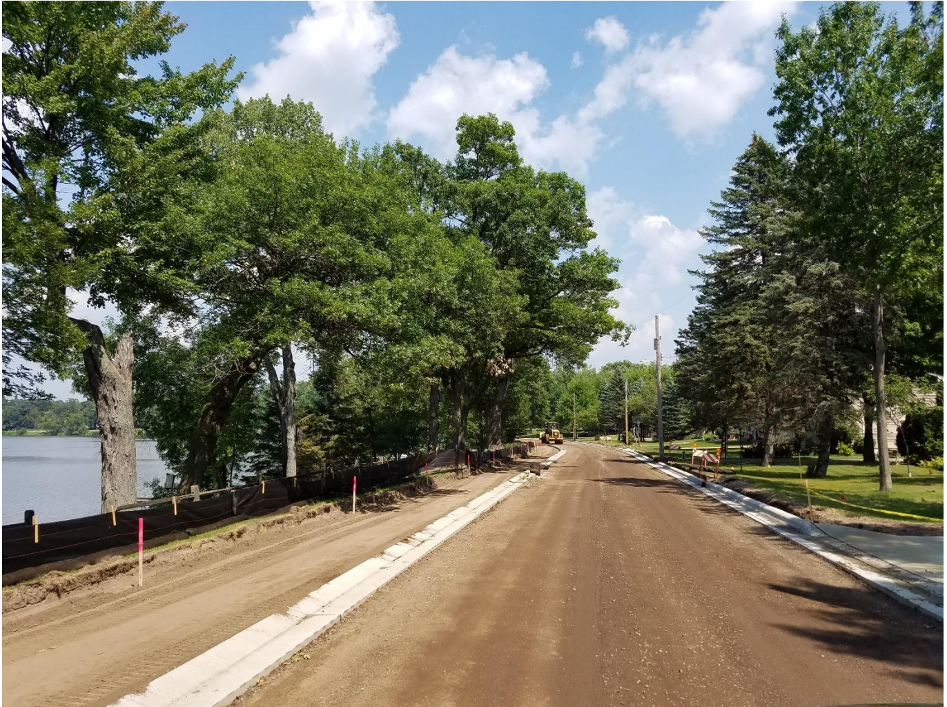
Concrete curb and gutter was recently placed on Birch Lake Boulevard South. The road and trail are scheduled for paving early next week!
