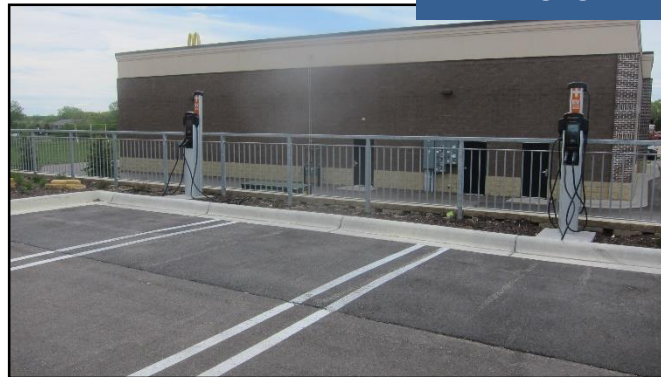
EV Charging stations
