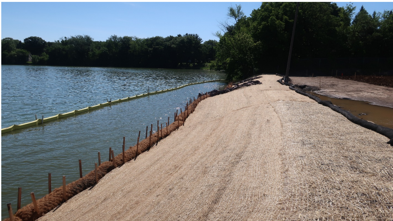
June 12, 2020 – Shoreline after grading, seeding and installation of temporary erosion control blanket (looking east)
