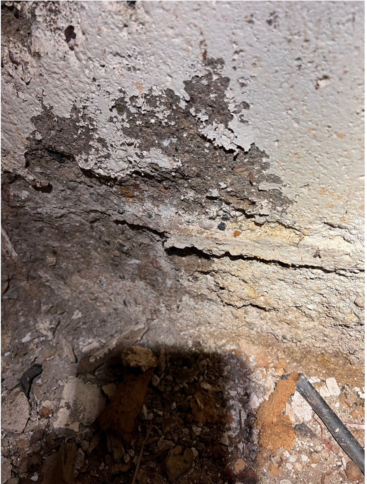
12-Interior basement foundation water damage
