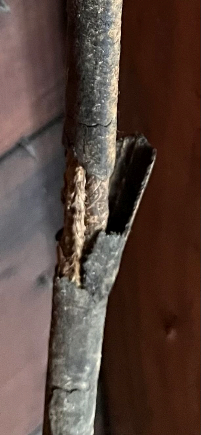
1- Electrical 1- decay of cloth insulation
