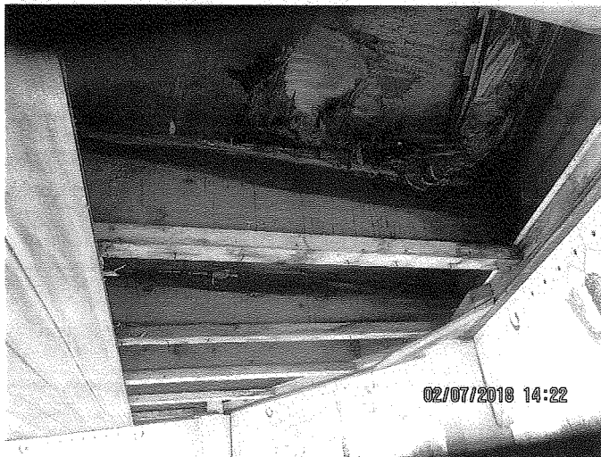
Photograph 3 Rotted floor joists
