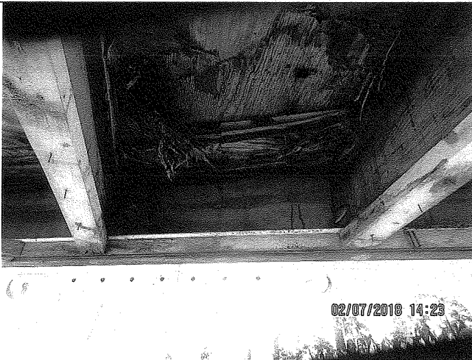
Photograph 5 Rotten floor sheathing
