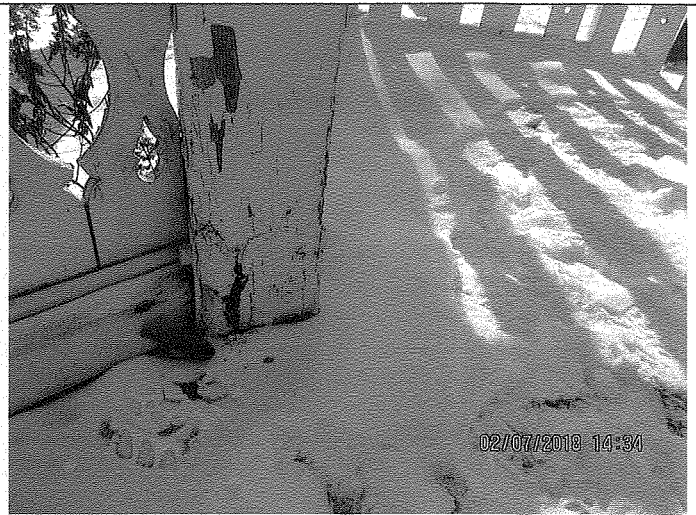
Photograph 6 Rotten bottom 6-inches to 1-foot of wood columns
