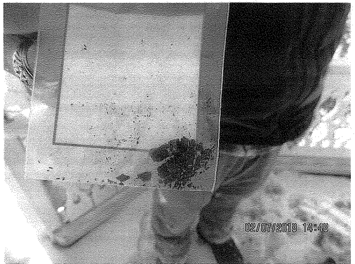
Photograph 8 Rotten wood from sample Number 2
