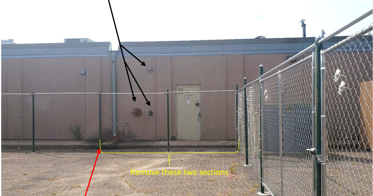
Recommended extent of fenced area – approximately in line with down-spout. (Photo taken from north facing south)
