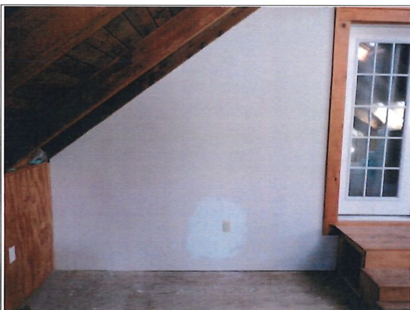
17 Existing conditions along north side of upper level loft area over garage.
